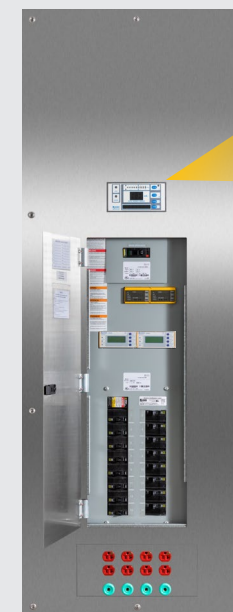
Bender's isolated power system (IPS) Panel
