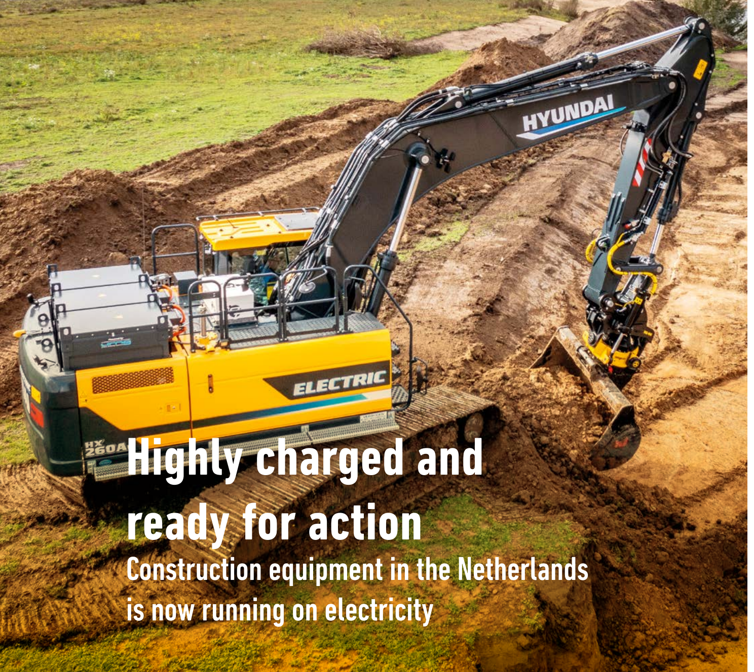
An electric excavator hard at work: The power supply is provided by three replaceable battery packs.
