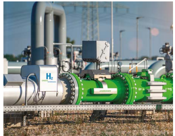
Green hydrogen needs sustainably generated electricity. Bender ensures that PV fields, for example, are electrically safe.
