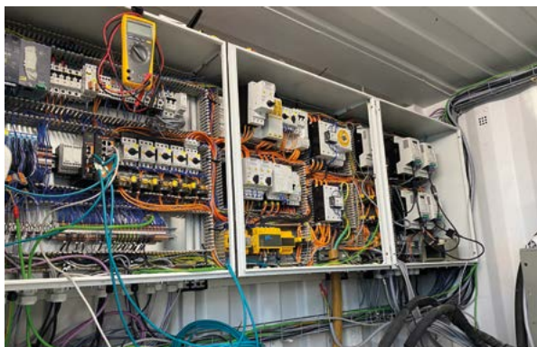
Control cabinet of tunnel boring technology with Bender components.
