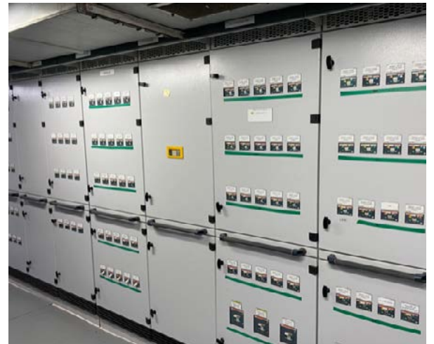
The emergency switchboard with the monitored load groups makes it easier to locate faults.
